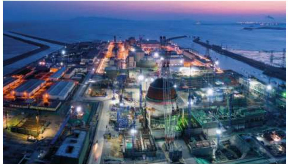
Fuqing power plant (Image: CNNC)
